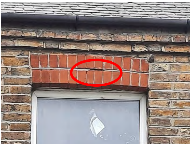
Plate 4.26: Gap within the Brickwork Above the Window
