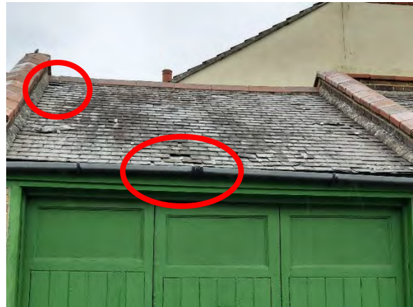
Plate 4.5: Missing and Lifted Roof Tiles
