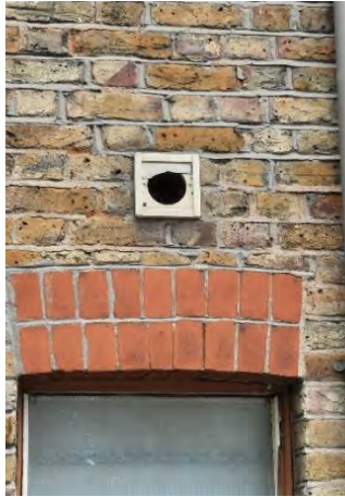
Plate 4.28: Gap in the External Wall
