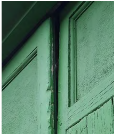
Plate 4.15: Gap Where the Garage Door is Ajar
