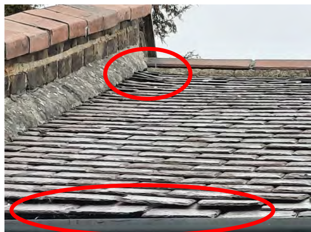
Plate 4.7: Lifted Roof Tiles
