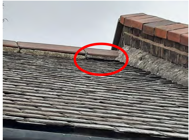
Plate 4.9: Gap Underneath the Ridge Tile
