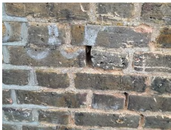
Plate 4.12 Gap Within the Brick Wall
