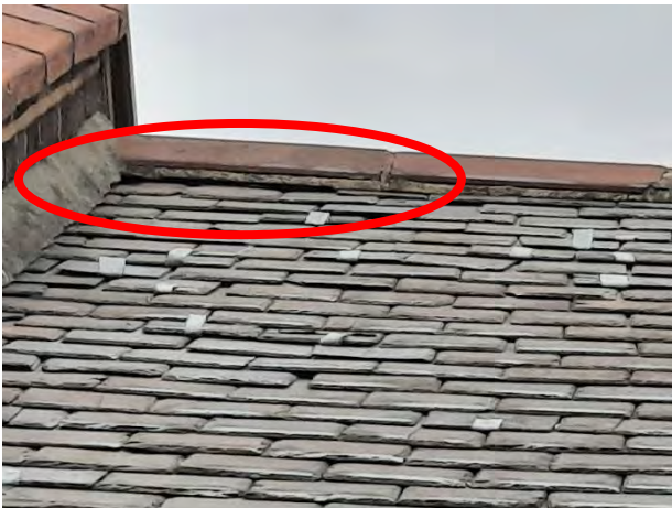
Plate 4.10: Gap Underneath the Ridge Tile
