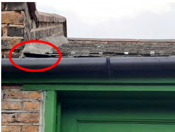
Plate 4.6: Lifted Roof Tile
