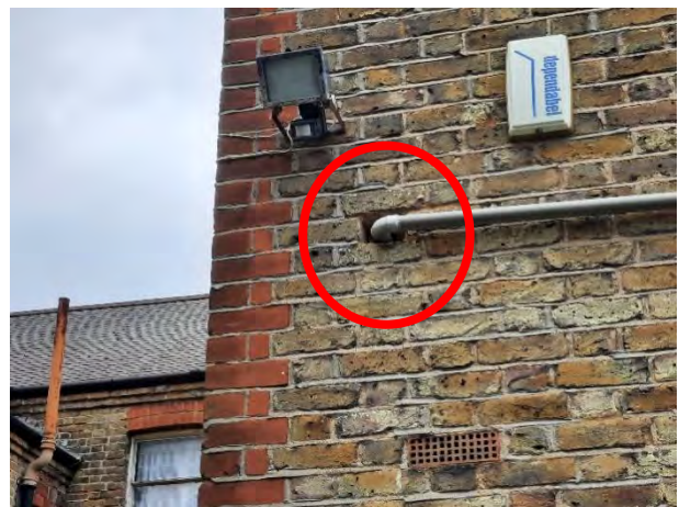
Plate 4.27: Gap Around the Pipe
