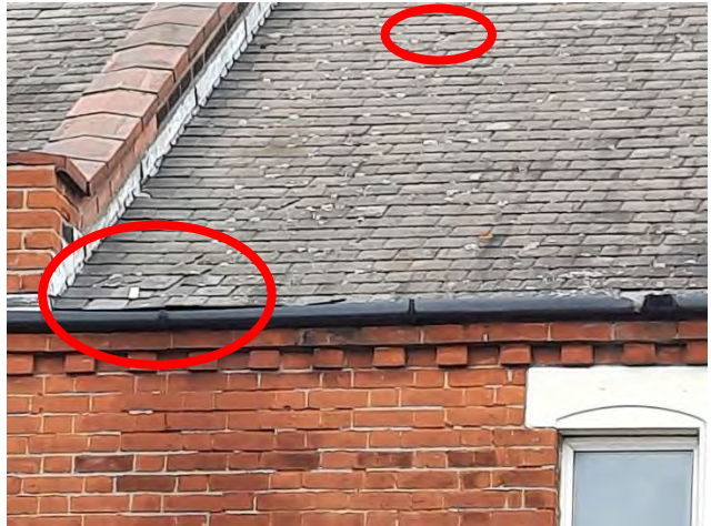
Plate 4.24: Slipped Roof Tiles
