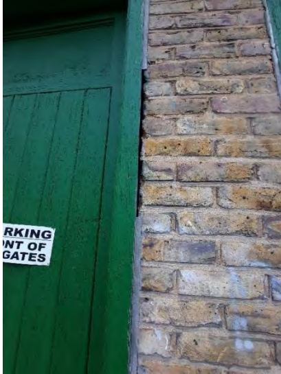
Plate 4.13 Gap Between the Wall and the Garage Door
