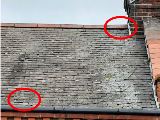
Plate 4.23: Damaged Tile and Gaps Under Tiles
