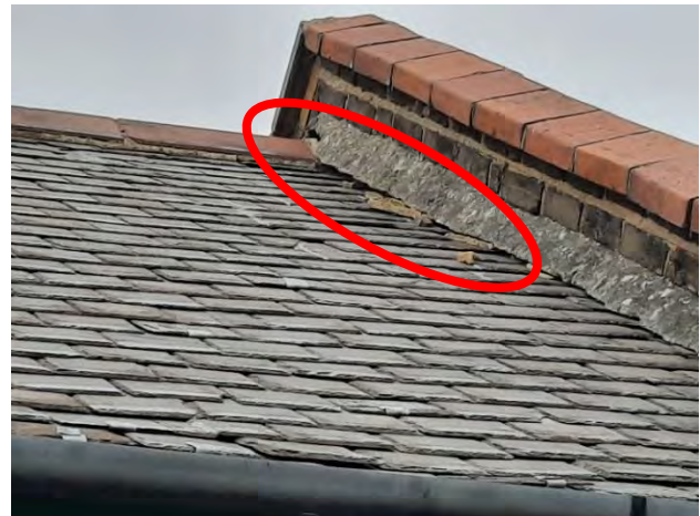
Plate 4.11 Gap Underneath the Cement
