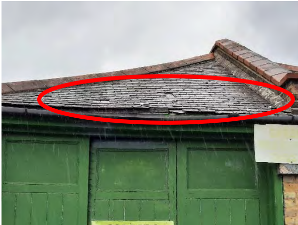
Plate 4.4: Missing and Slipped Roof Tiles
