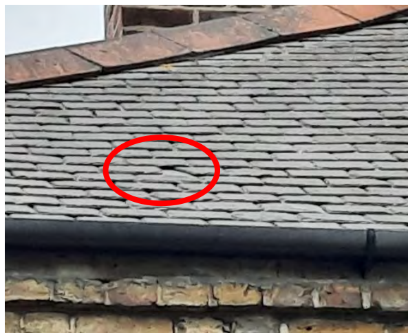
Plate 4.25: Slipped Roof Tile
