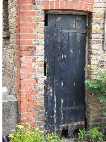
Plate 4.29 Gaps Within the Door
