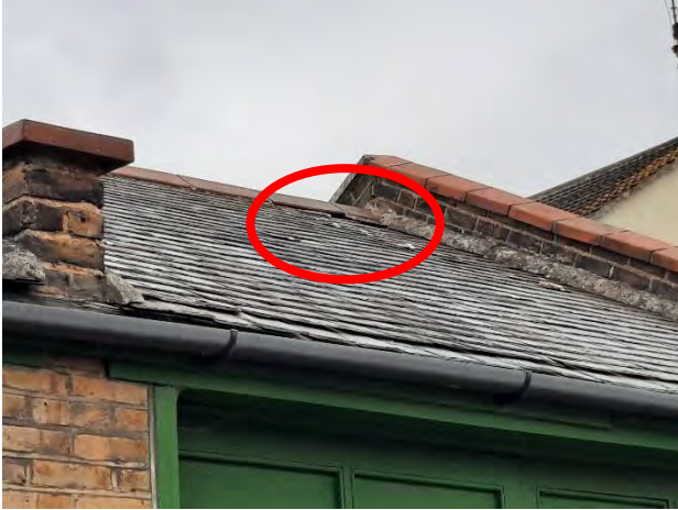
Plate 4.8: Gap Underneath the Ridge Tile
