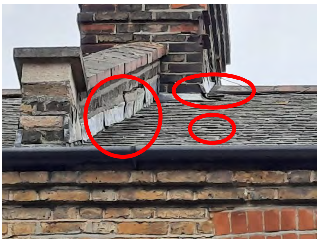
Plate 4.22: Lifted Lead Flashing and Gap Under a Tile
