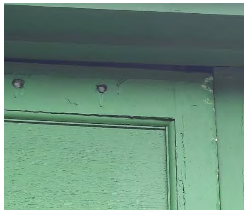
Plate 4.16: Gap Where the Garage Door is Ajar
