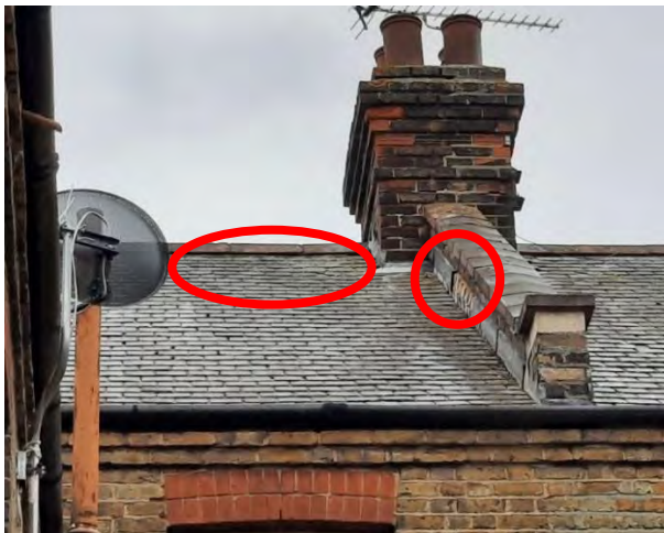
Plate 4.21: Gap Under Ridge and Lifted Lead Flashing
